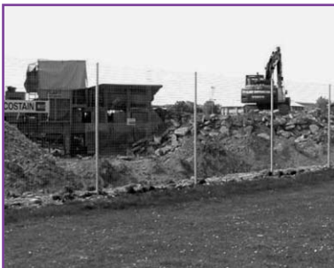
Removing the old concrete from the former RAF runway in warm dry weather caused much dust. The concrete was broken up and used in other foundations
